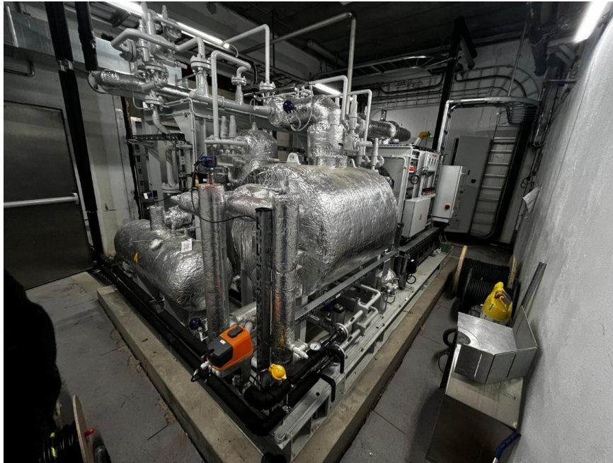
Figure 3. Mayekawa's Ammonia heat pump installed at Stella Polaris' site
